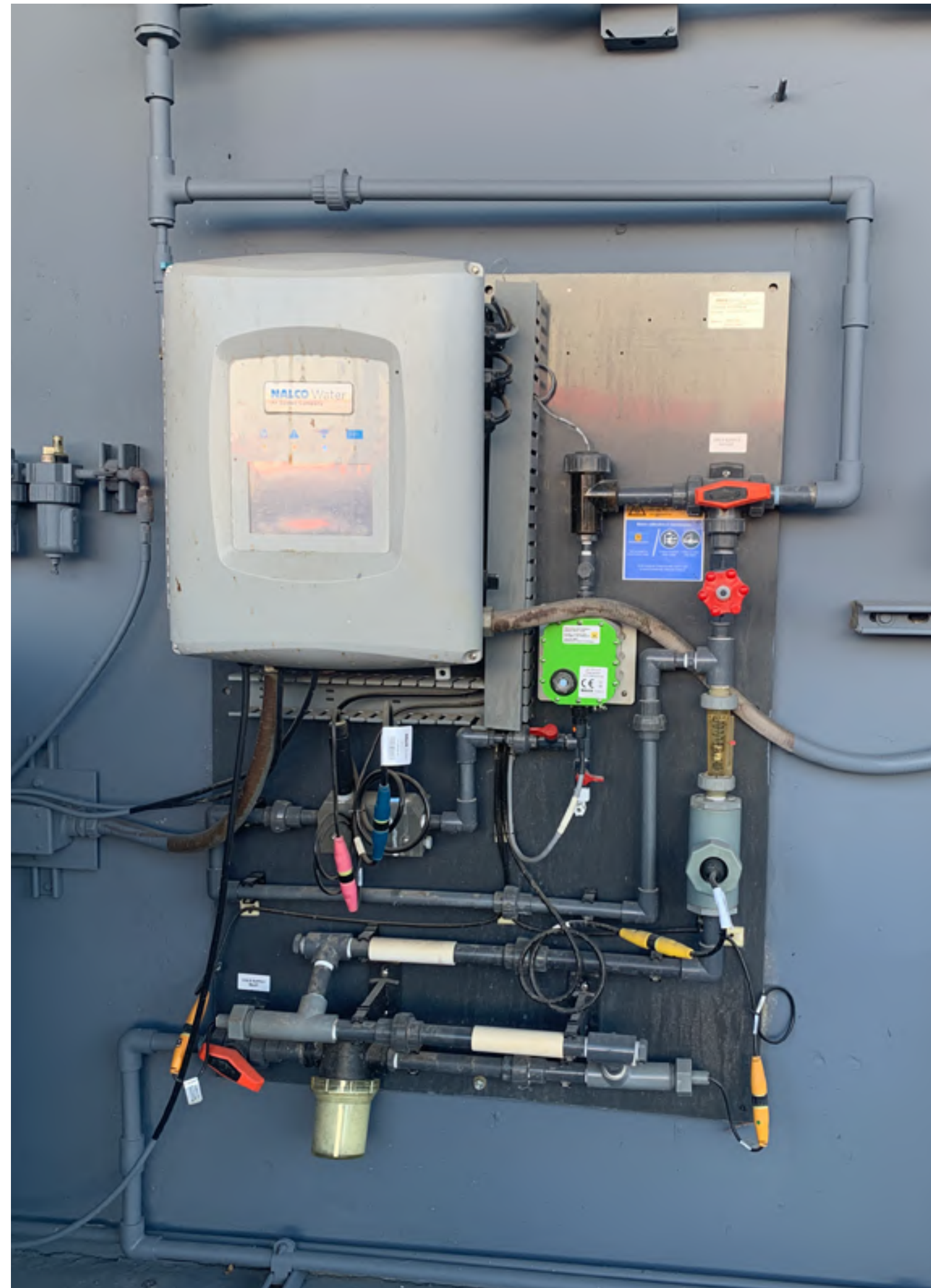
Cooling Tower Tempe, Ariz
